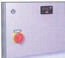
Front view of a cabinet with the display unit, easily visible, mounted on the front of the door, whilst the protector unit is installed deep within
