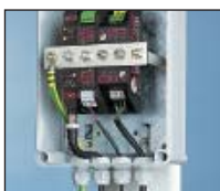
Protectors for the video (ESP CCTV/B, left), camera telemetry (ESP 06E, centre) and the low current mains power (ESP 240-5A, right) inputs to a camera, installed together on a CME 4 mounting and earthing kit. Note that the protectors have been cross bonded to the metal work of the pole (out of shot)
